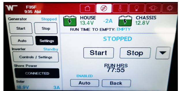
Generator Settings Screen
